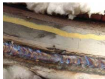
Fig. 6 — Crack in the heat-affected zone during initial repair.
