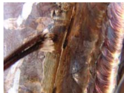
Fig. 5 — Crack in the weld during initial repair.
