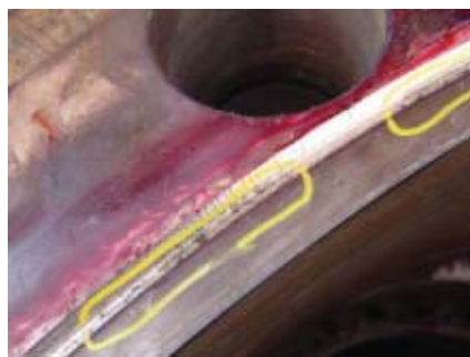
Fig. 2 — Cracks on the stainless steel cladding on the flange face.
