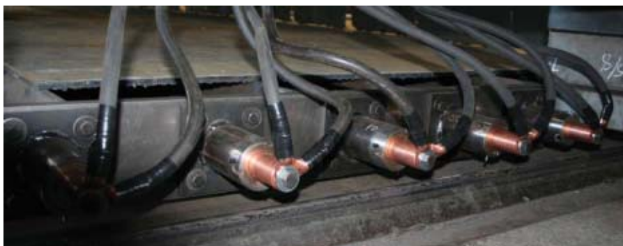
Fig. 4 — The back side of this system features a new 4/0 workpiece lead for each inverter and routes them two to a plunger.
