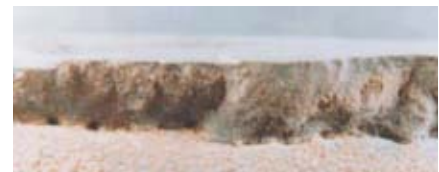
Fig. 3 — An example of a cold crack that has occurred in the toe of the weld (a toe crack). This type of crack initiated nearly parallel to the base metal surface and propagated from the toe of the weld where residual stresses are higher. (Photo from AWS B1.11, Guide for the Visual Examination of Welds.)
