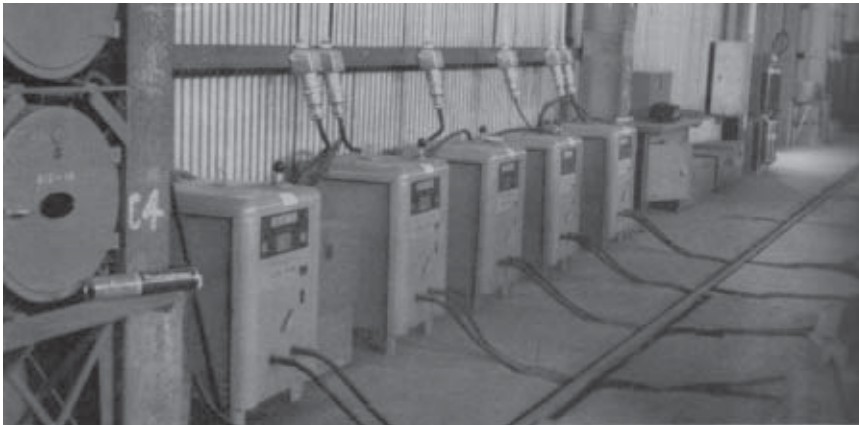
Fig. 4 — Typical installation of silicon rectifier arc welding units, which became popular during the 1960s. (From “Silicon — The Key to a Reliable Welding Power Source” by Lewis F. Petit, which appeared in the the November 1961 Welding Journal.)
